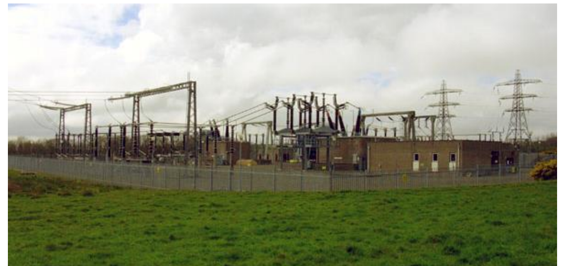
Alverdiscott National Grid substation
